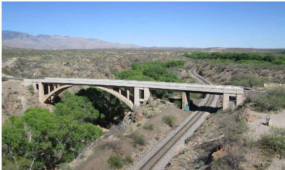
Cienega Creek Bridge in Pima County's Cienega Creek Natural Preserve, built in 1920-21 and listed on the National Register. (Photo: $1LENCE)
